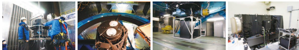
Figure 1: (a) [Left] PFI being lifted from the test bench on the floor in the telescope area for the installation into POpt2 later. (b) [Middle left] PFI after the installation on the prime focus of the telescope. (c) [Middle right] MCS installed on the telescope at the Cassegrain focus. (d) [Right] SM1 operating in the dedicated temperature-controlled clean room inside the telescope dome building to receive photons from the sky through PFI and Cable B1.
