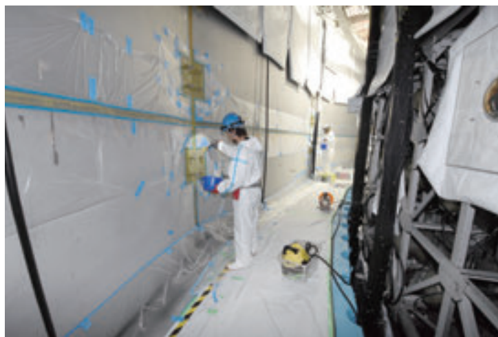
Figure 5: Sealant work on the SK tank wall being conducted from the floating floor. An outer detector PMT can be seen at the right side.
